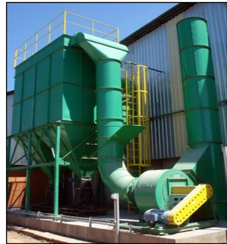
Fig. 12: Exaustor filtro manga
